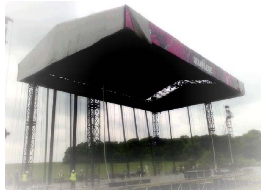
Download 2008, A-TECH supplied fit and telehandler operators, climbers and steel hands for the build and derigs
